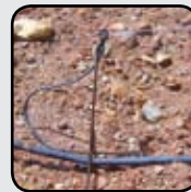
Ore-Max Sprinkler Systems: Custom designed systems for the pad.
